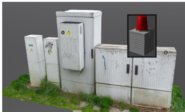
Fig. 2. Outdoor Cabinet and Alarm System
