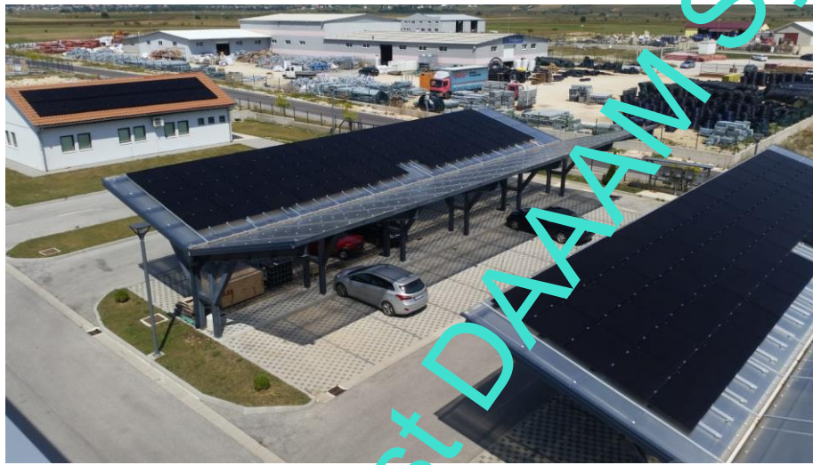
Fig. 3. 50 kW PV plant in Tomislavgrad [3]
