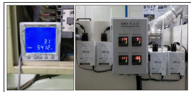
Fig. 2. Electric power meter and temperature controller
