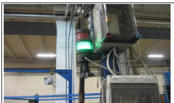
Fig. 4. Control lamp for welding process
