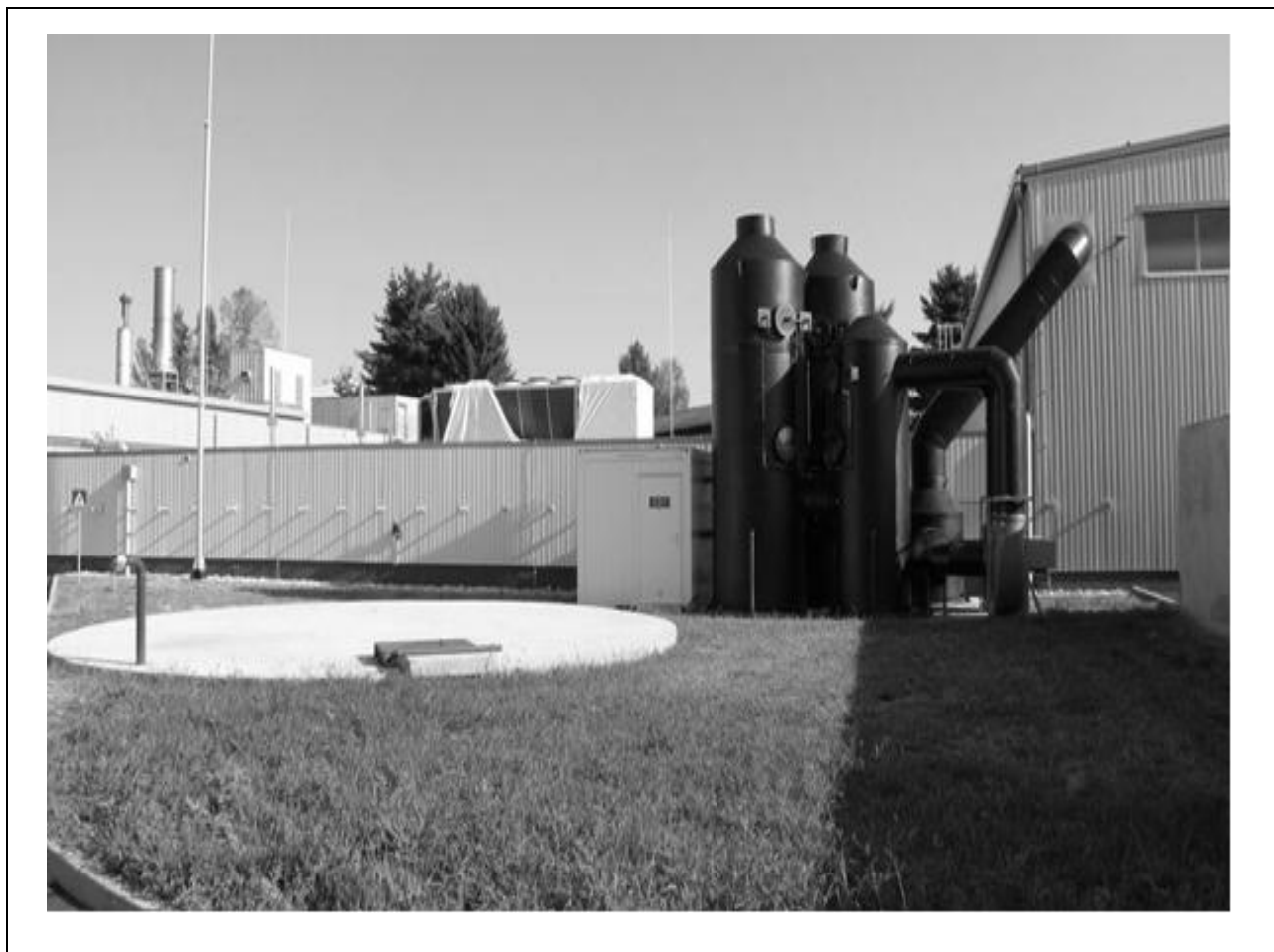
Fig. 3. Two horizontal fermenters of the biogas plant Drazenci
